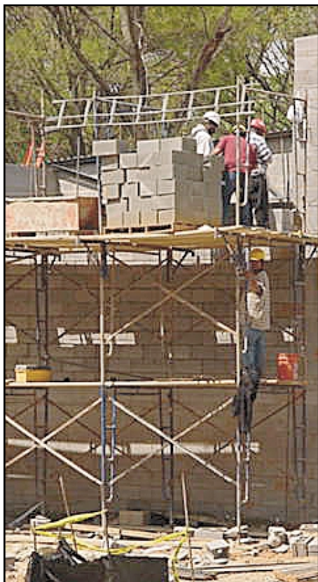
There was no spring break last week for crews building tomorrow's schools. At the new Merry Oaks Elementary (above), parts of the roof are on toward a scheduled January opening date. The $12.4 million project off Central Avenue was financed by '97 school bonds.
