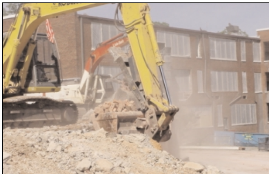
Dust flies at Elizabeth Elementary off Park Drive as demolition workers finish clearing a one-story annex last week, part of an $11.3 million renovation of the 1925 building and construction of new space. The school is meeting at old Druid Hills until the scheduled August 2003 reopening.
