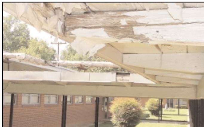
A canopy at old Barringer Elementary shows its age. Voters will be asked in November to approve a bond issue for $224 million to expand and renew CMS schools, and build new ones to keep up with growth.
